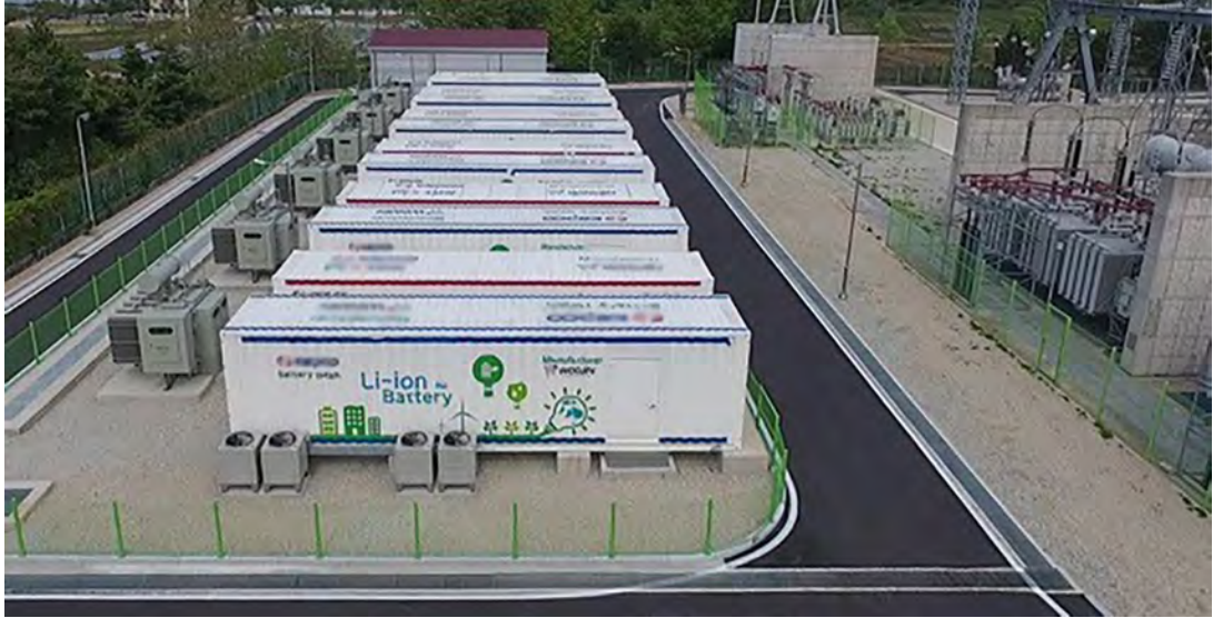
Figure D.4: Sokcho Battery Energy Storage System
